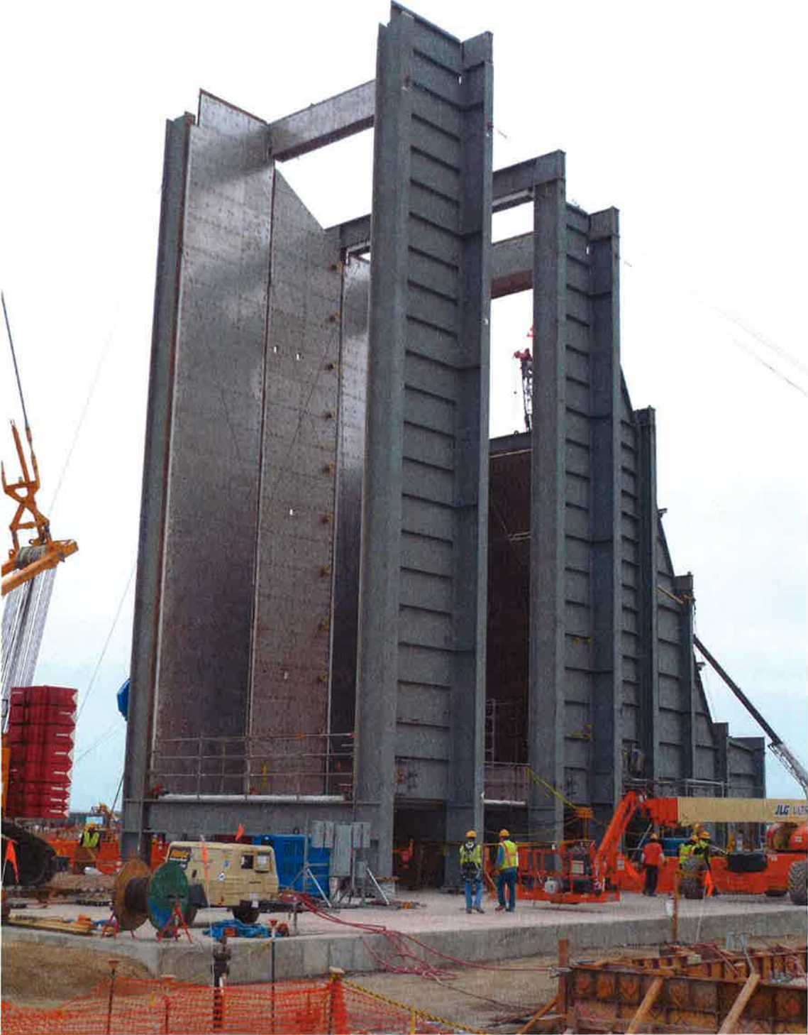
Photograph #3 HRSG #1 Framing, Showing the Locations of the High, Intermediate, and Low Pressure Sections
