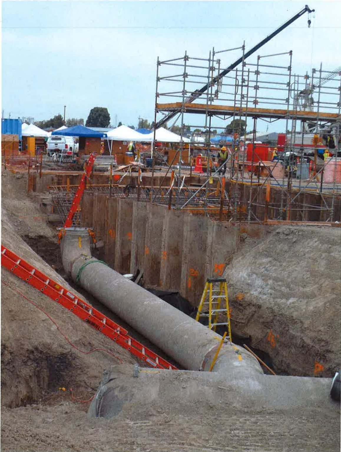
Photograph #4 Piping in open trenches running between condenser and cooling tower
