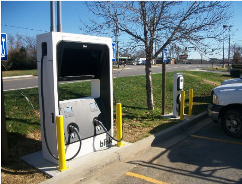
Figure 54. DC fast charging Installation 226
