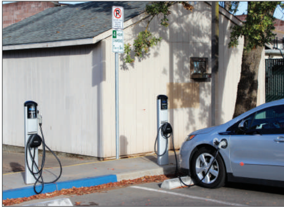
ChargePoint charging stations in the City of Sonoma, with signage and an ADA accessible parking spot.
