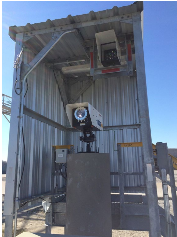
Figure 17. Example of a UV-DOAS analyzer installation.
