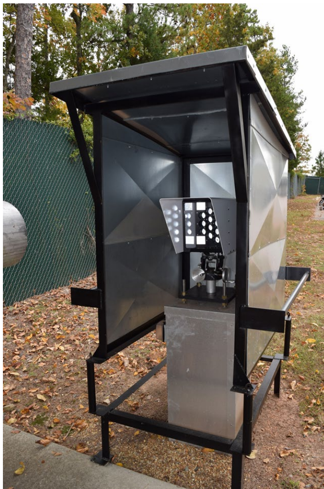
Figure 18. Example of a UV-DOAS retroreflector installation.
