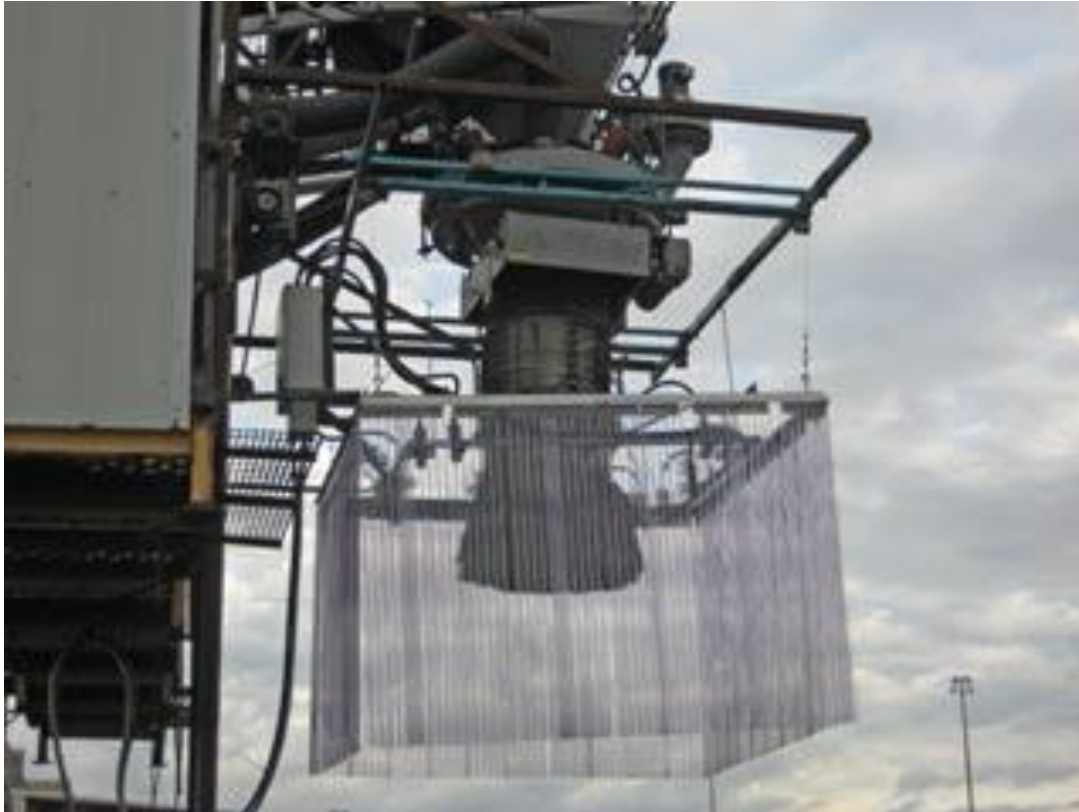
Figure II-3: Wind Barrier surrounding a transfer point
