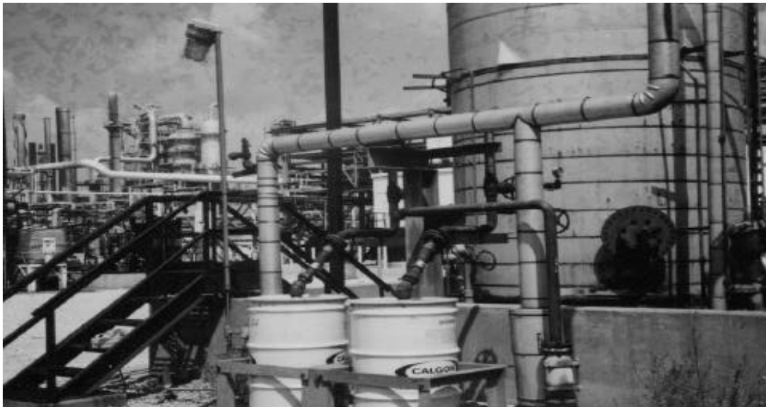
Figure 4 Use of Carbon Adsorption for Control of Wastewater Collection Systems at a Refinery 10
