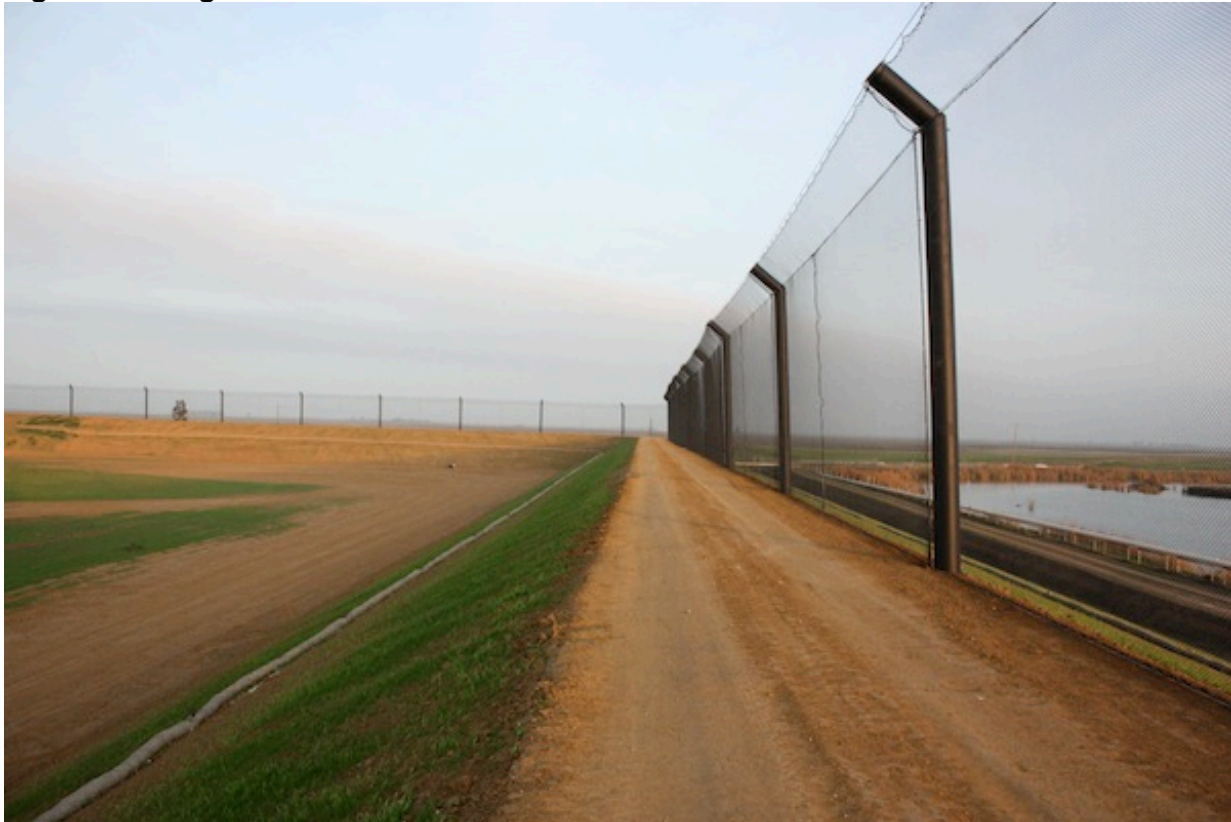
Figure II-7: Fugitive Dust Control with Wind Screen
