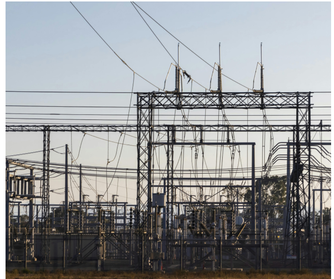
Power Distribution Substation (Creative Commons)
