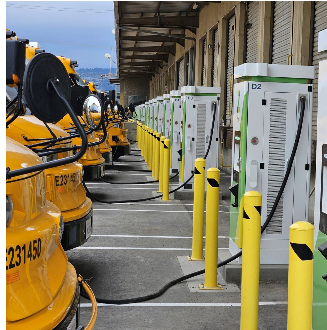
Source: Air District equipment inspection
