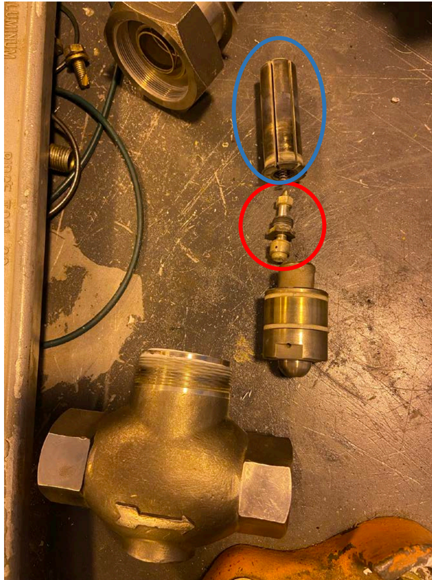
Figure 3: Deconstructed Aktomatic Solenoid Valve. The plunger, circled in red, periodically unthreads from the plunger housing, circled in blue. During annual preventative maintenance, the mechanic applies sealant to the plunger's threads.
