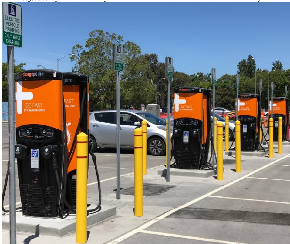
Figure 7. Eight DC Fast Chargers Installed at the NASA Ames Visitor Center Parking Lot
